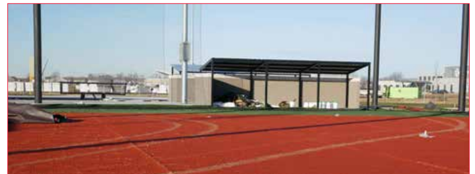
Construction at the Greenwood Sports Park continues ahead of its opening in 2024. (Photo courtesy of City of Greenwood)
