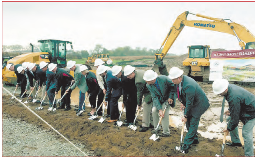
School officials and developer Lancer + Beebe, LLC, break ground on Walnut Grove Elementary. (Photo by Nicole Davis)
