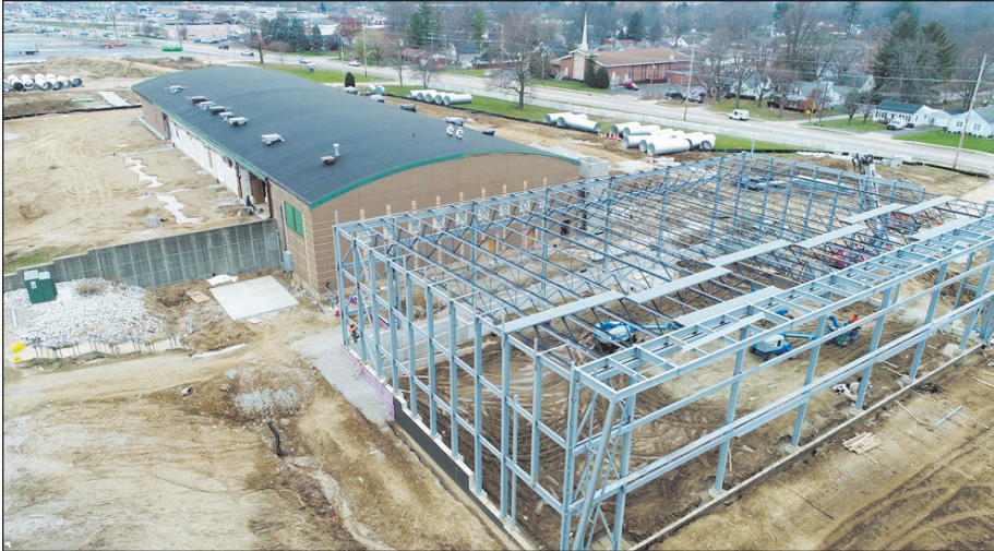
Progress continued on construction of the future Greenwood fieldhouse, expected to be completed this year. (Submitted photo)
