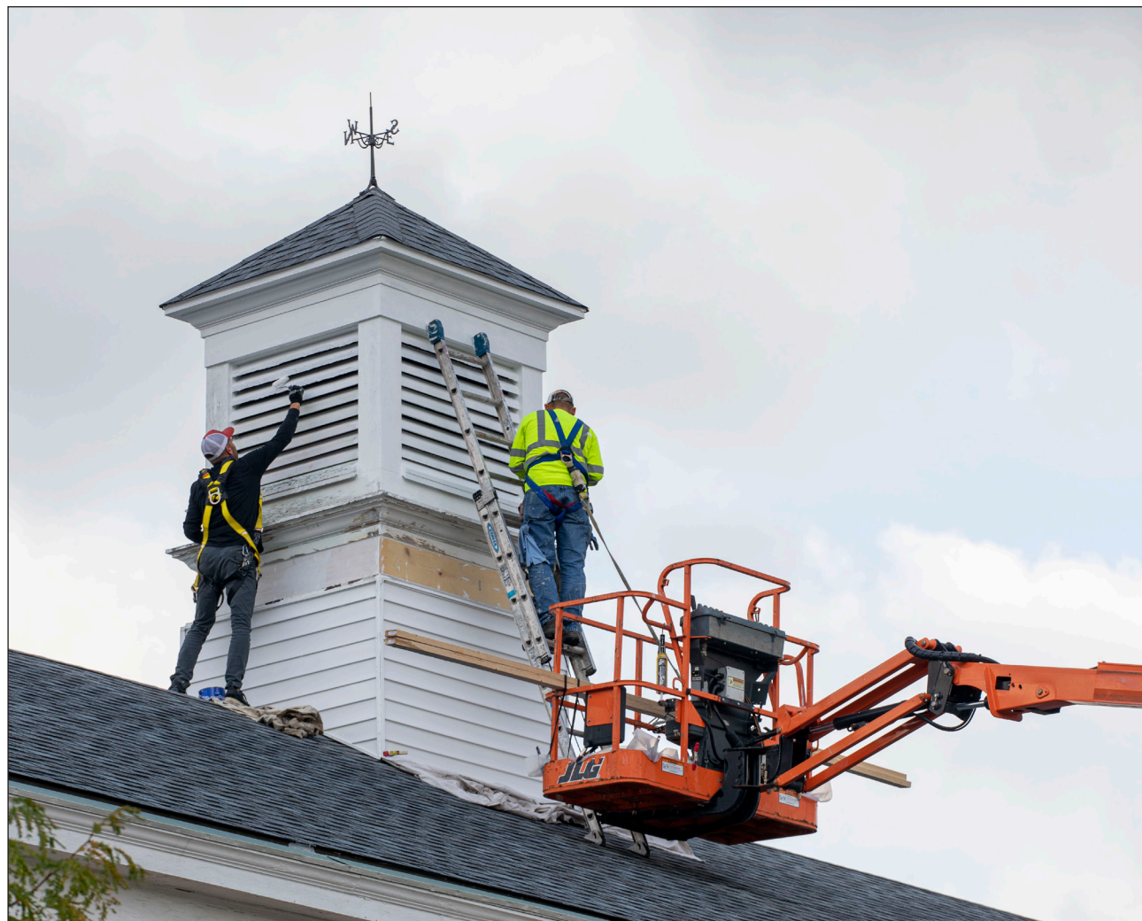
City employees work on painting the spire on top of the Post Office building Oct. 21, 2021, on Main Street in Beech Grove. The repainting work at the post office is one of many things on Main Street that have been refurbished by the city. (Photo by Jacob Musselman)
