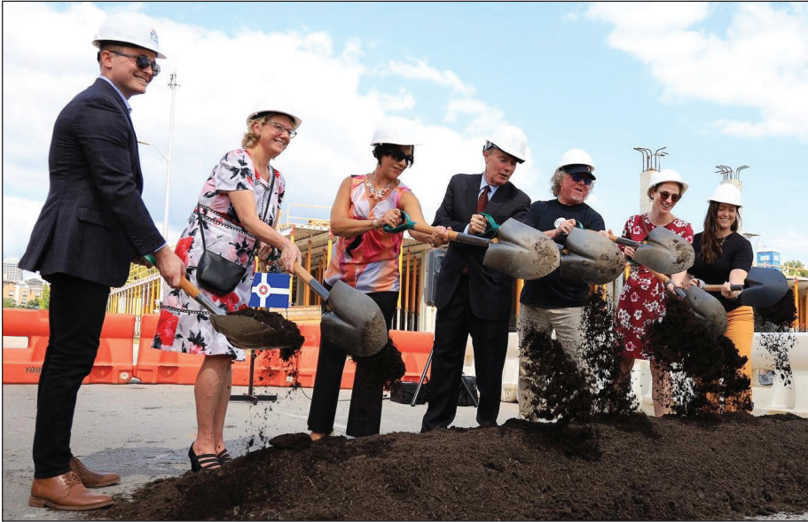
The city of Indianapolis and Old Southside community members celebrate the groundbreaking on South Meridian Street. (Photo by City of Indianapolis)
