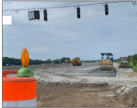
A view of the I-69 construction at Fairview Road. (Photo by Nicole Davis)
