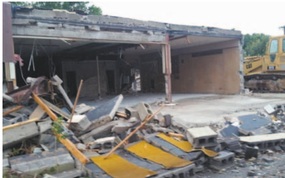
The WTTV-4 building on Bluff Road was demolished this month. Photo by Laura Brown Hinton
