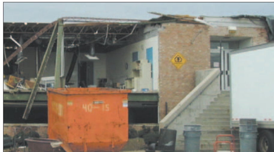
Above and below: Damage inside the Baxter YMCA after tornado on Sept. 20, 2002. Submitted Photos
