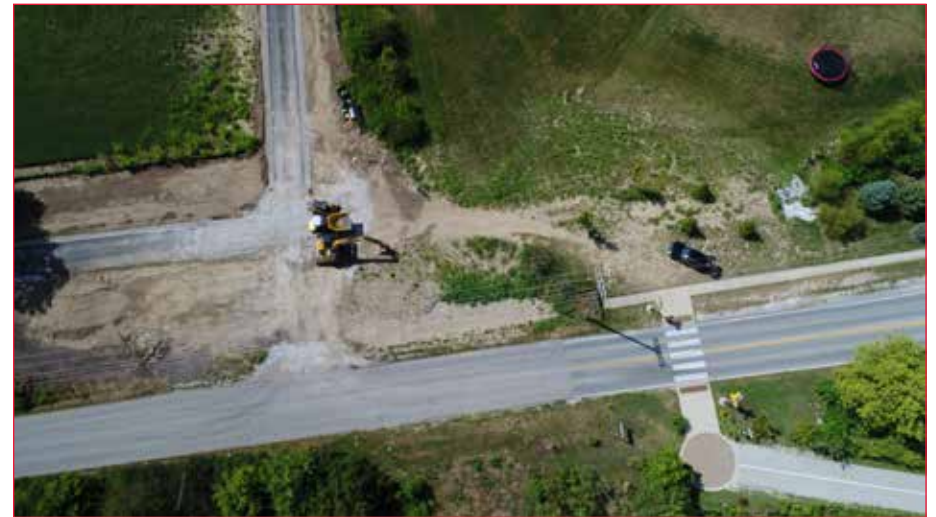
Aerial view of the Bicentennial and B&O Trail under construction in Brownsburg.
