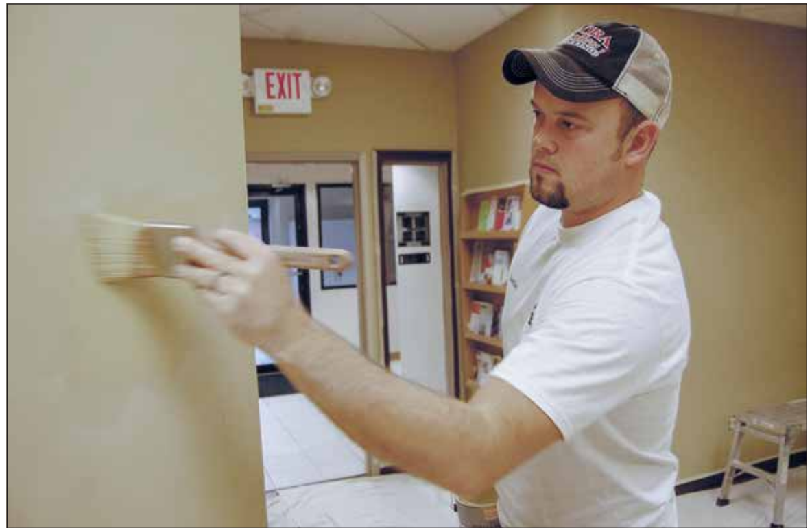
Justin Flora puts paint onto a wall at Susie’s Place, Avon, in December of 2015. The Flora Brothers have embraced Hendricks County - and giving back is paramount to their business model. (Photo by Rick Myers)
