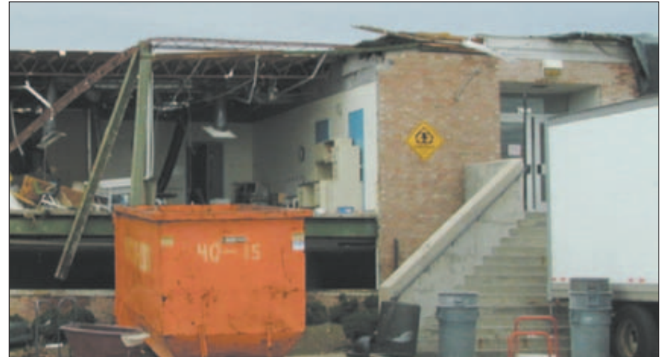
Above and below: Damage inside the Baxter YMCA after tornado on Sept. 20, 2002. Submitted Photos
